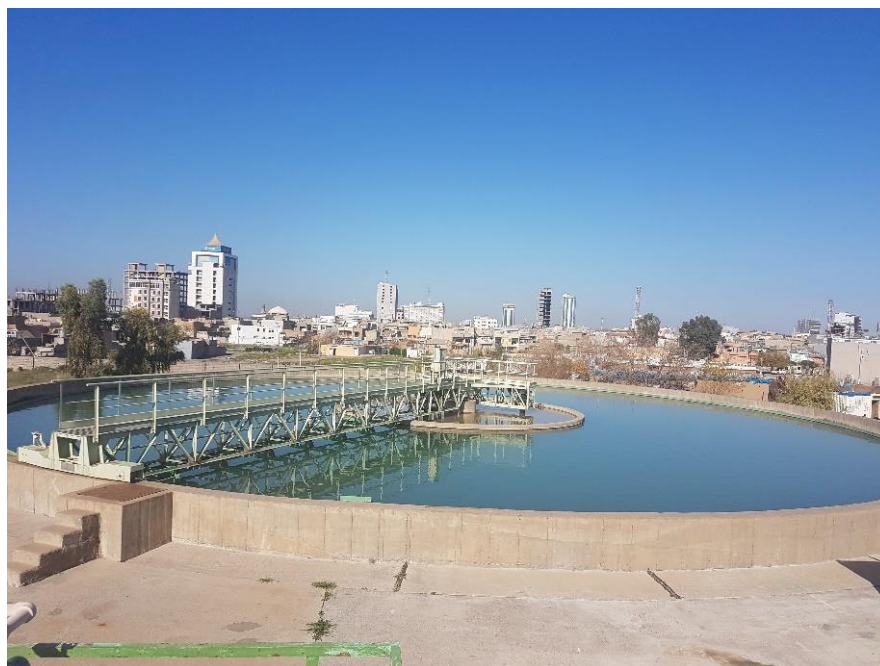
Figure 5: Sedimentation tank with flocculation unit
