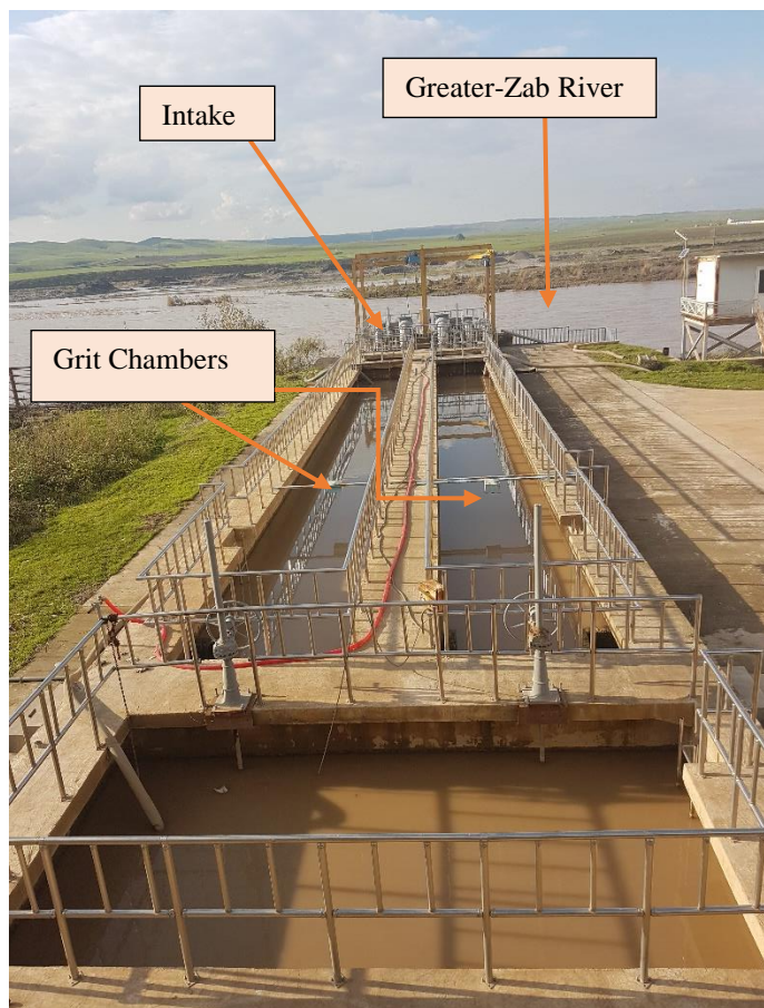
Figure 4: Water intake of Ifraz 2 (WTP) on Greater-Zab River
