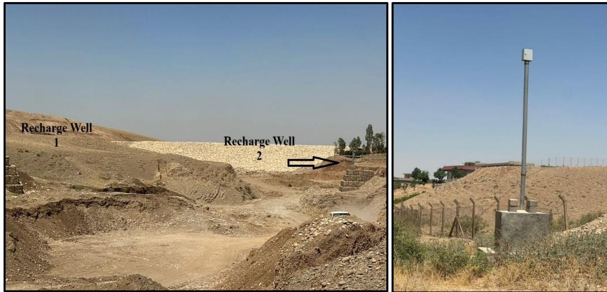
Figure 2: Two recharge wells and one monitoring well at the Tarin pilot site (Captured on Jun 22, 2025)
