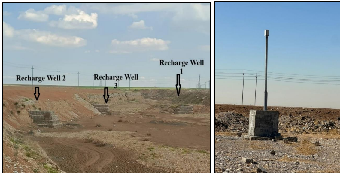
Figure 4: Three recharge shallow wells and one monitoring well at the Daratoo pilot project site (Captured on April 17, 2025)
